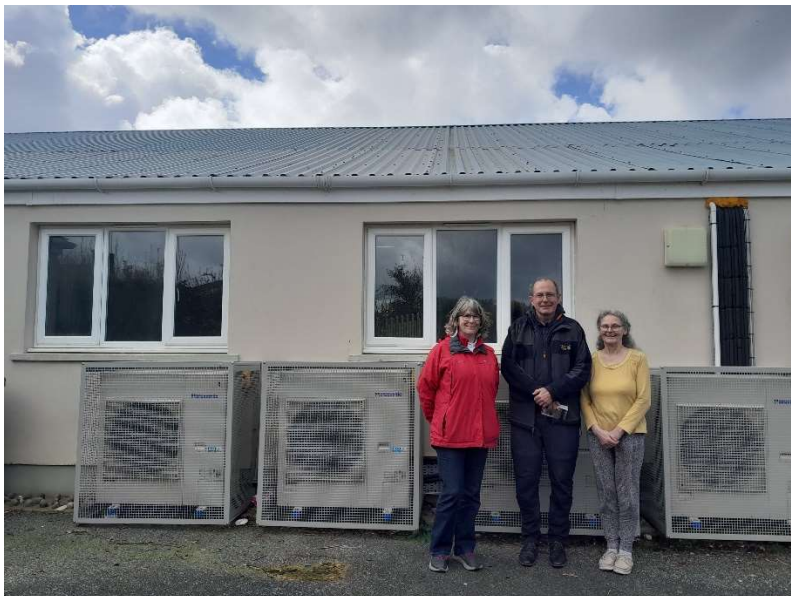
From left to right, Kate Hawkins, the TBG link person for Letterston Hall, Mike Davies, TBG Trustee and volunteer, and Babs by the external fans which extract heat from air outside the hall.
