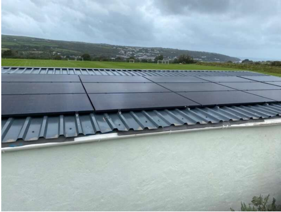
The solar PV array at the Football Club
